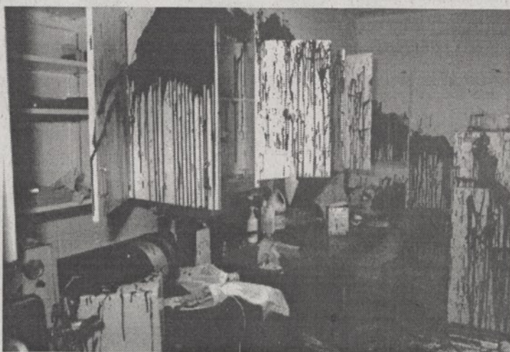
Extensive damage inside the laboratory room.
